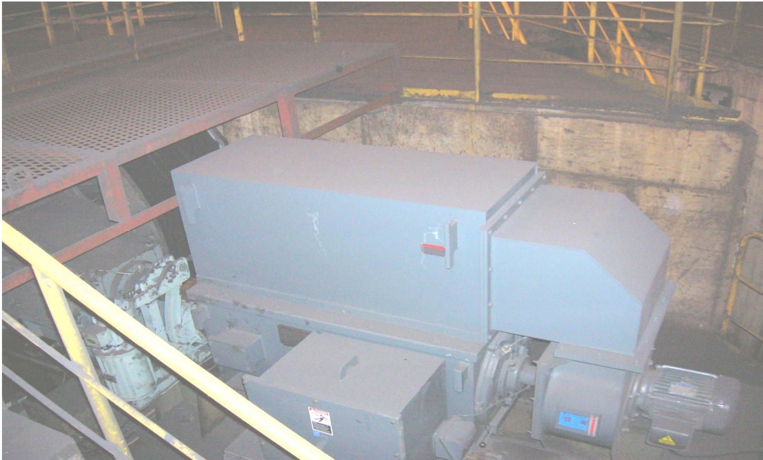
260KW 6P VECTOR INVERTER MOTOR (4 units)
